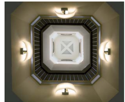
VIEW OF RESTORED CUPOLA FROM TIERED LOUNGE AT SECOND FLOOR BELOW - AFTER
