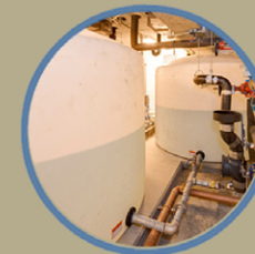
Cisterns with Ozone Circulation
