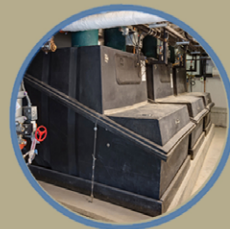
Composting Toilet Tanks
